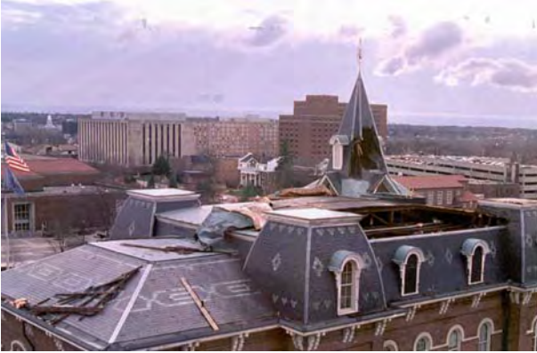
This was the view from the Liberal Arts and Education Building on December 7, 1998. A windstorm the night before tore off the roof, which struck the cupola as it lifted away. Photograph by David Umberger.
