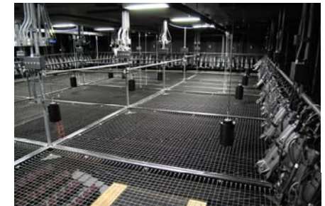
The suspension grid, lighting storage and power distribution systems of the Mallett Theatre.
